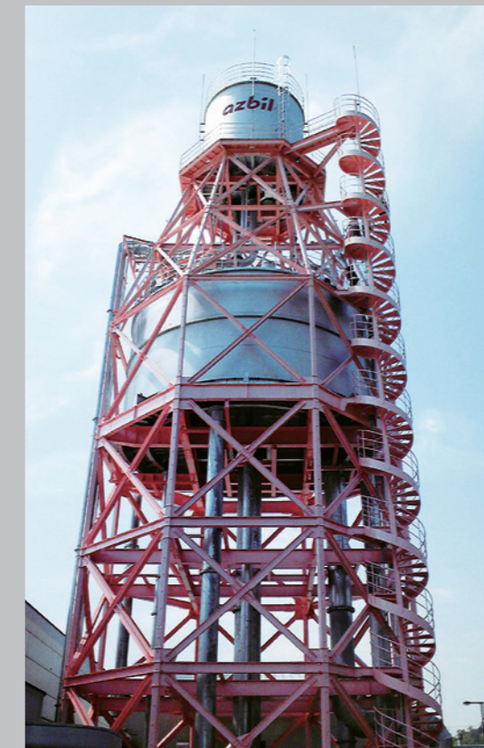
Elevated water tank for calibration
